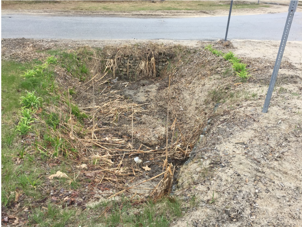
Photo 9. Landscape island at the intersection of Letter S Road and Frank C Gilman Hwy. Shallow depression conveys stormwater from the road and fire station to Outfall 10.
