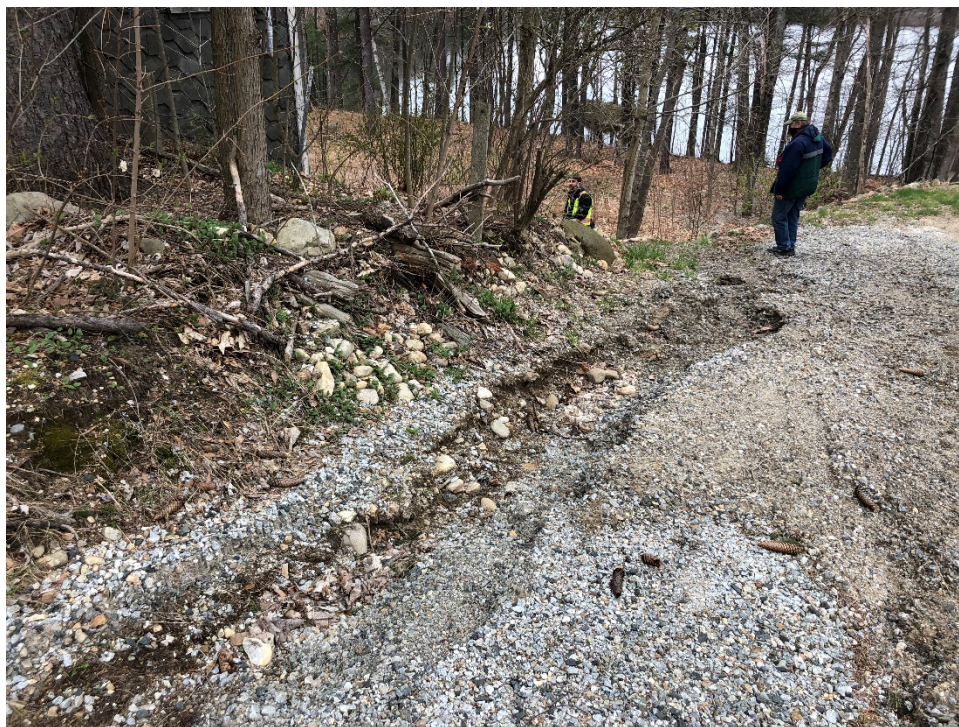
Photo 6. Severe channel erosion down the driveway of 189 Main Street towards Mill Pond.
