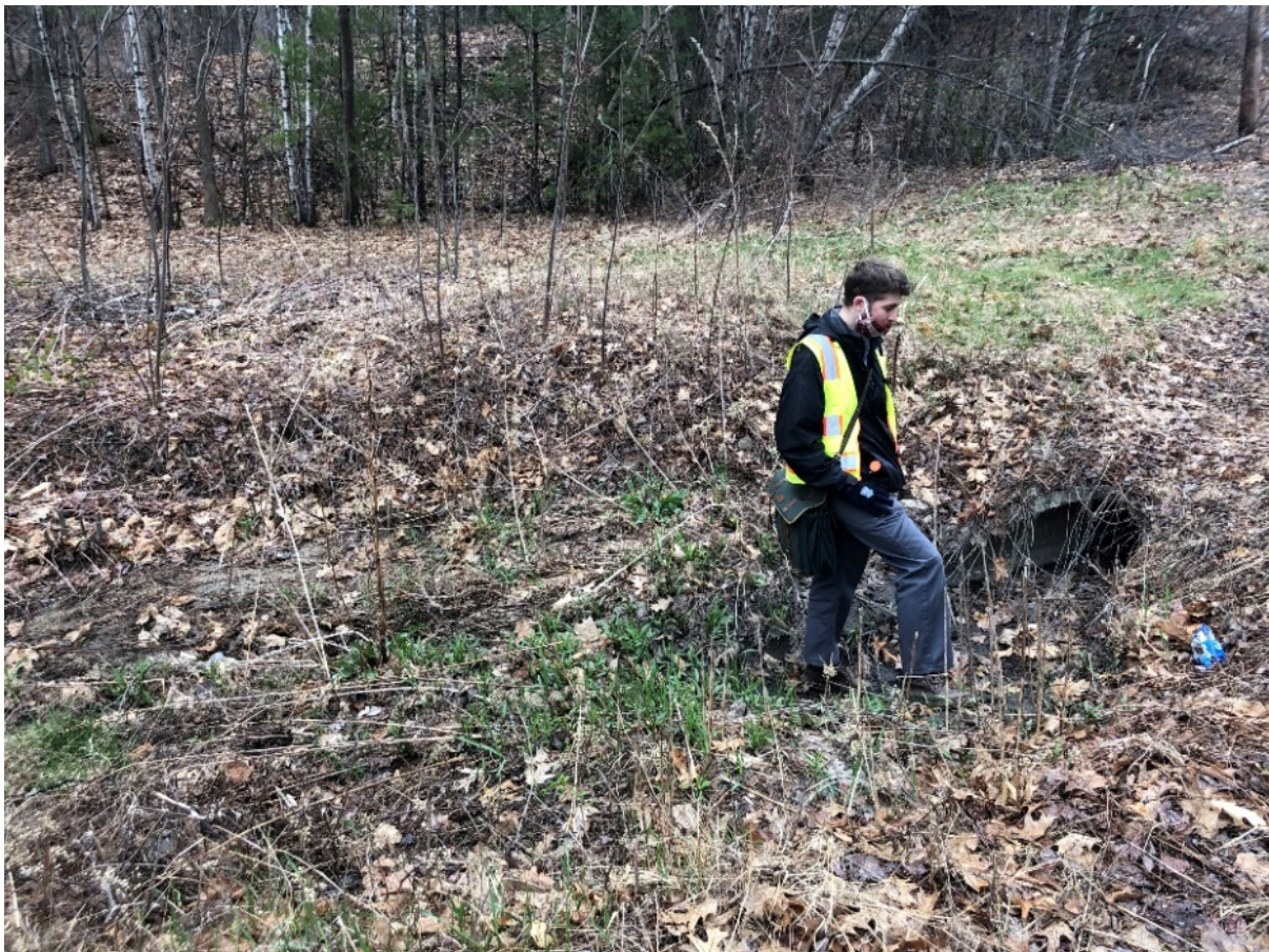
Photo 1. Outfall 1 is clogged with leaves and is set lower than the swale leading to Mill Pond.
