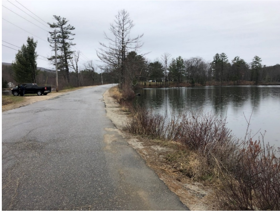
Photo 12. Bank instability and erosion along Letter S Road.
