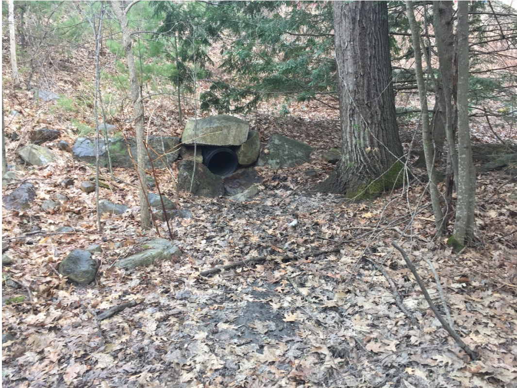
Photo 7. Outfall 6 discharging into shallow depression.
